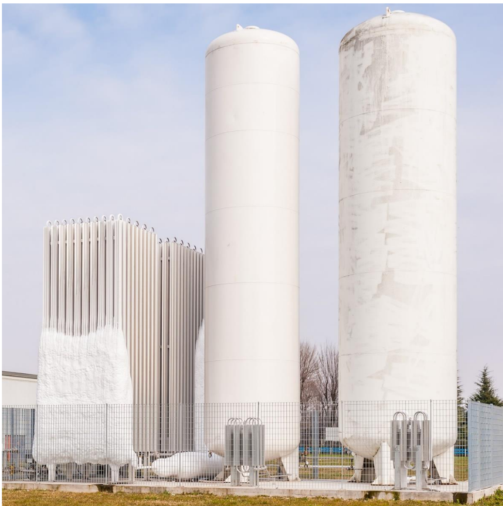
Picture no. 19: Cryogenic tanks.
